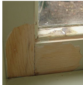
Stained and damaged window at master tub
