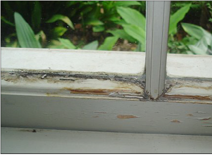
Rotted wood with slight mold growth at north master bedroom bay window
