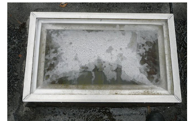
Moisture in bathroom skylight
